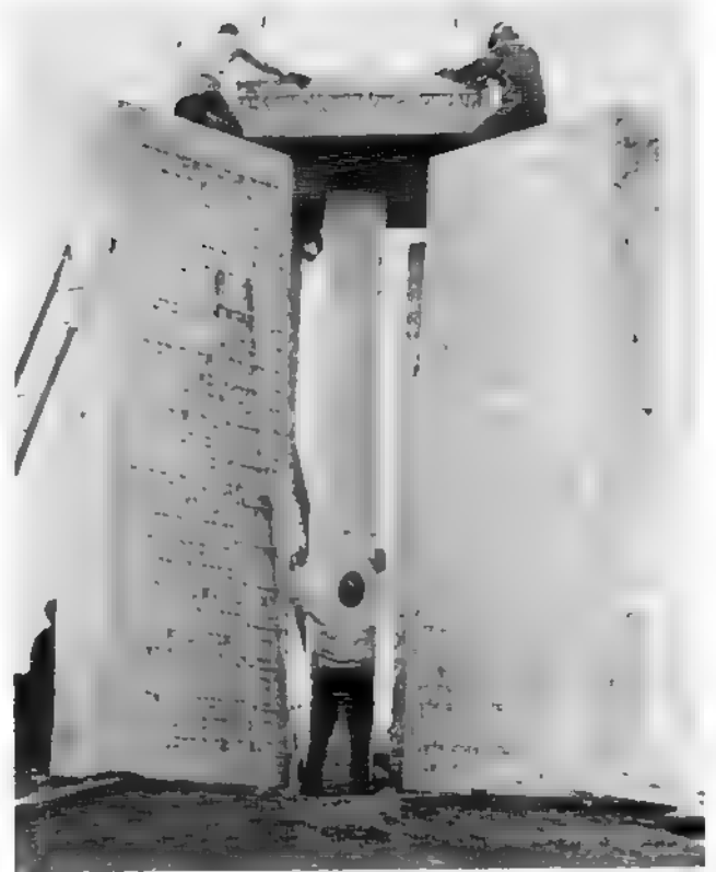
During the waning twilight of March 12, 1980 the final section, the large capstone, was set into place to complete construction of The Georgia Guidestones . Joe Fendley, builder, is shown directing placement of the capstone. All that remained to be done was steam-cleaning the stone for the March 22nd dedication.
